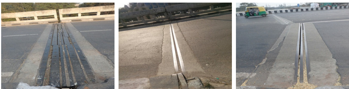
Fig: - Damaged Expansion joint Filled with debris
