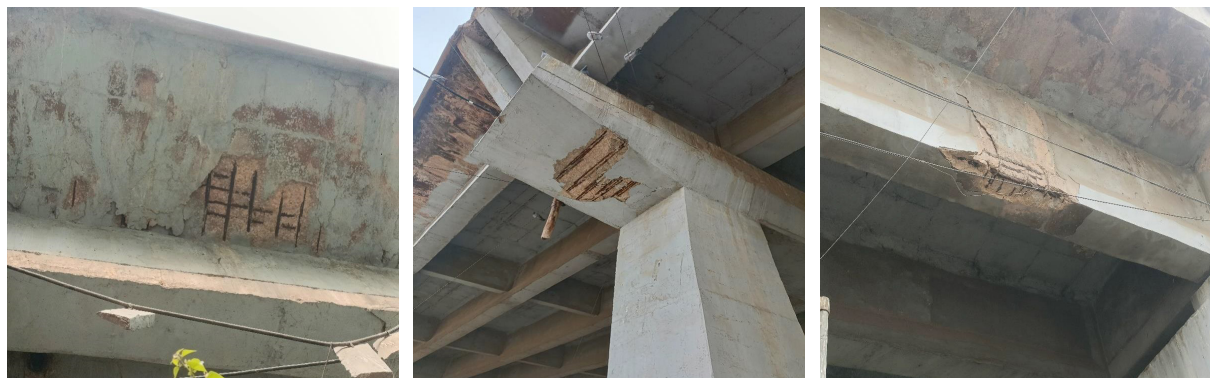
Fig: - RCC Spalling in Deck slab, Pier Cap & Girder
