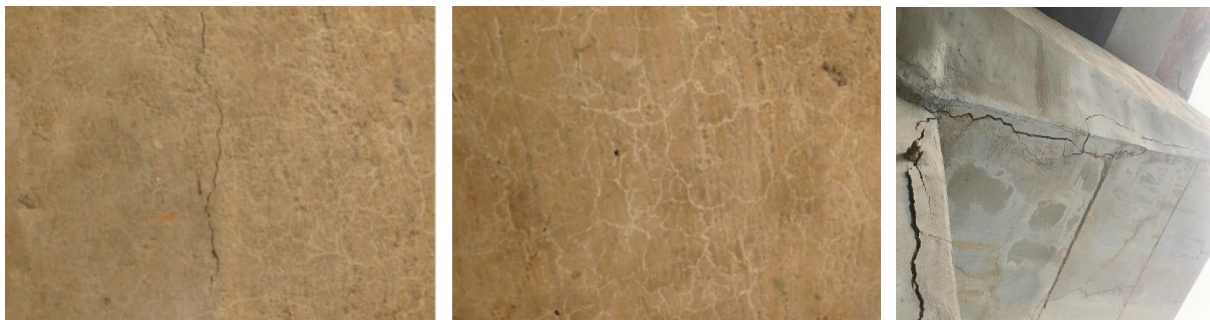
Fig: - Cracks in pier& pier caps
