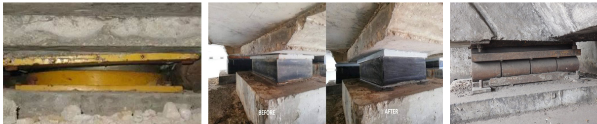
Fig: - Malfunctioning of Metal & Elastomeric Bearings
