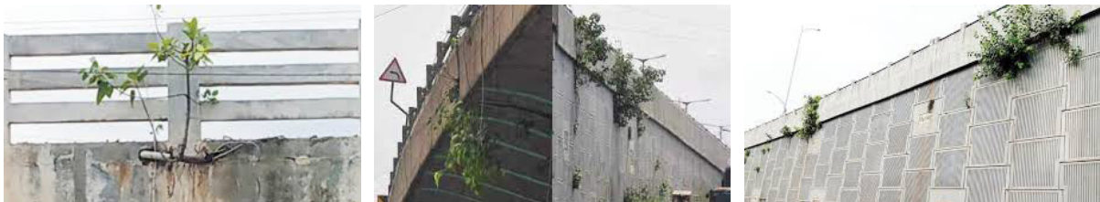
Fig: - Vegetation Growth in Retaining wall and Railing
