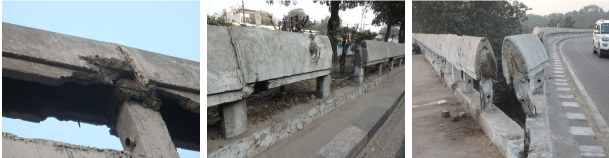
Fig: - Distressed Crash Barrier and RCC Railing
