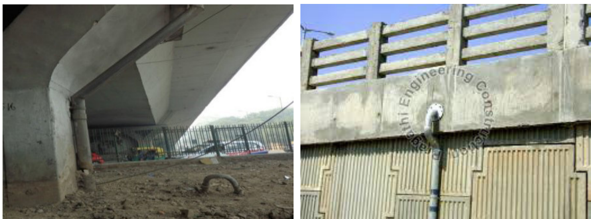
Fig: - Failure of drainage system
