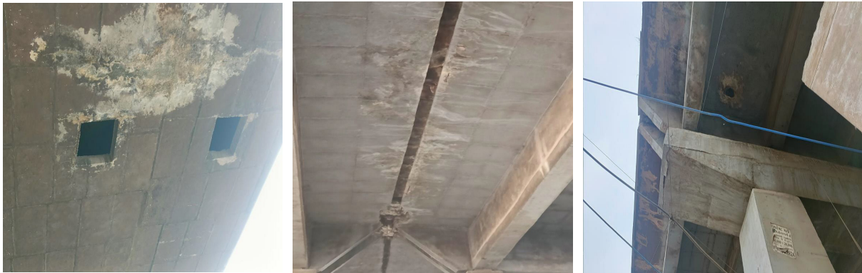
Fig: - Water Marks in Deck slab & Girder
